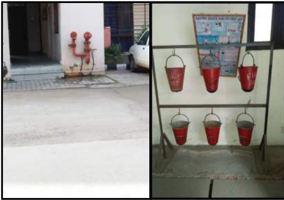
Fire Fighting Equipment
